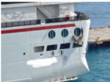
Figure 1 of 3 – Unsafe repositioning of a stage
