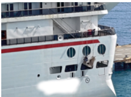
Figure 2 of 3 – Unsafe repositioning of a stage
