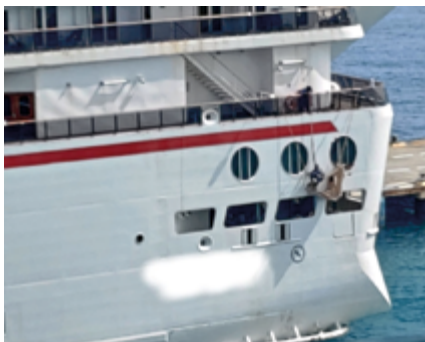
Figure 3 of 3 – Unsafe repositioning of a stage.
